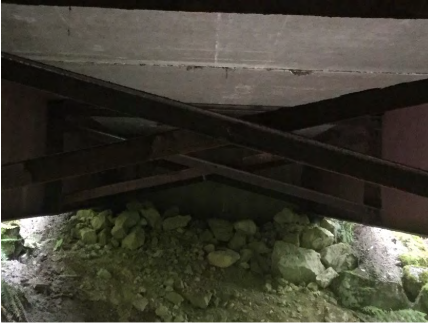
Some delamination of diaphragm occurring
